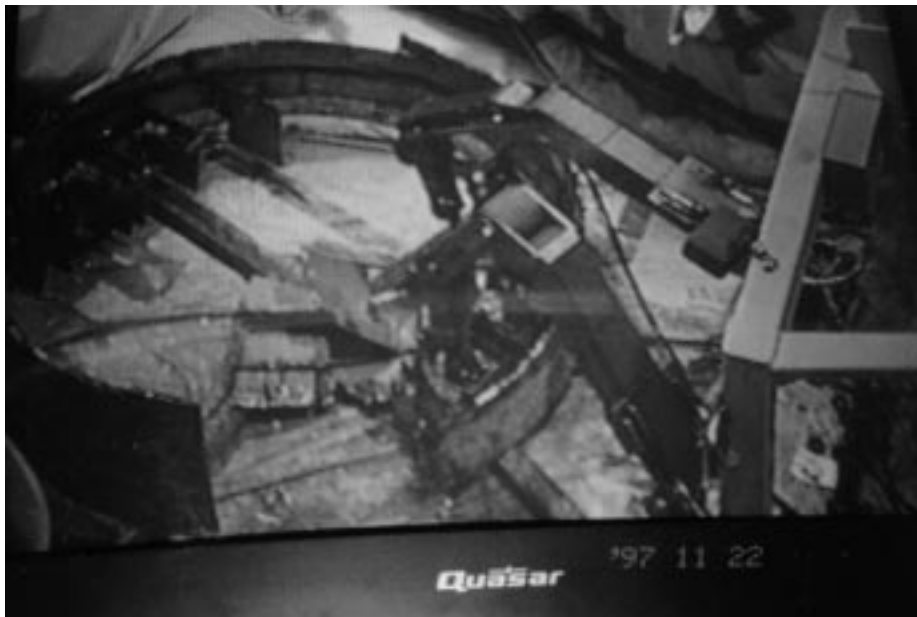
Figure 6. The View of Cutting Operations through Viewing Monitors from the Console Chair
