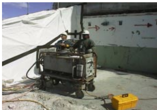
Figure 3. Electric/hydraulic power unit.
