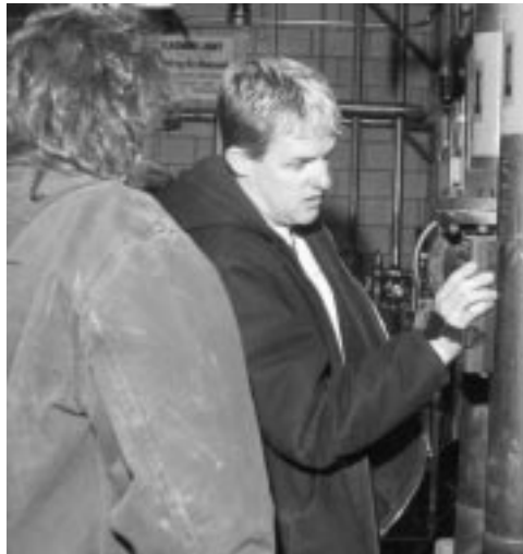
Figure 2. NITON® XL-800 Series Multi-Element Analyzer being used to analyze system piping
