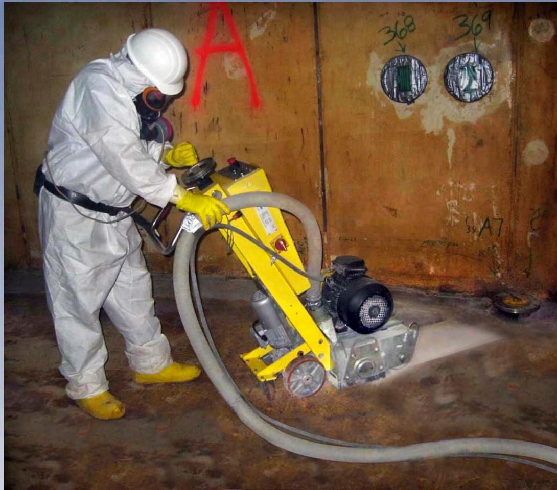
Diamond floor shaver being used to remove contaminants in Plum Brook Reactor decommissioning.
