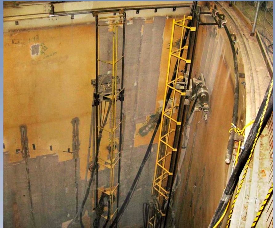
Diamond wall shavers with Bluegrass-engineered mountings removing contaminants from flat and concave walls at Plum Brook Reactor Facility.
