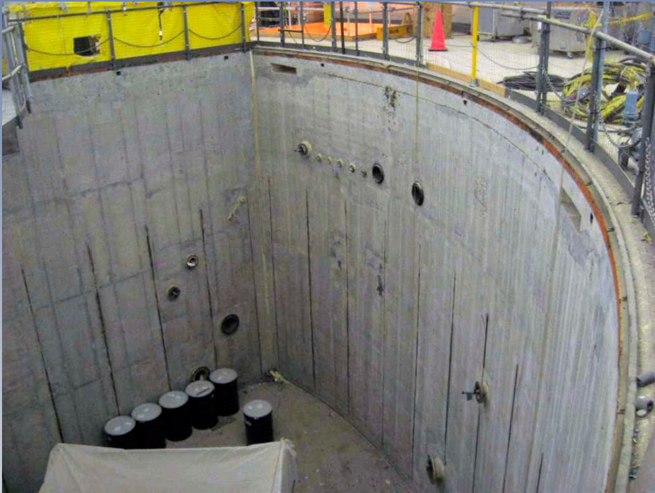
Finished walls and floors after contaminant removal. Waste is stored in 55-gallon drums at bottom of picture.
