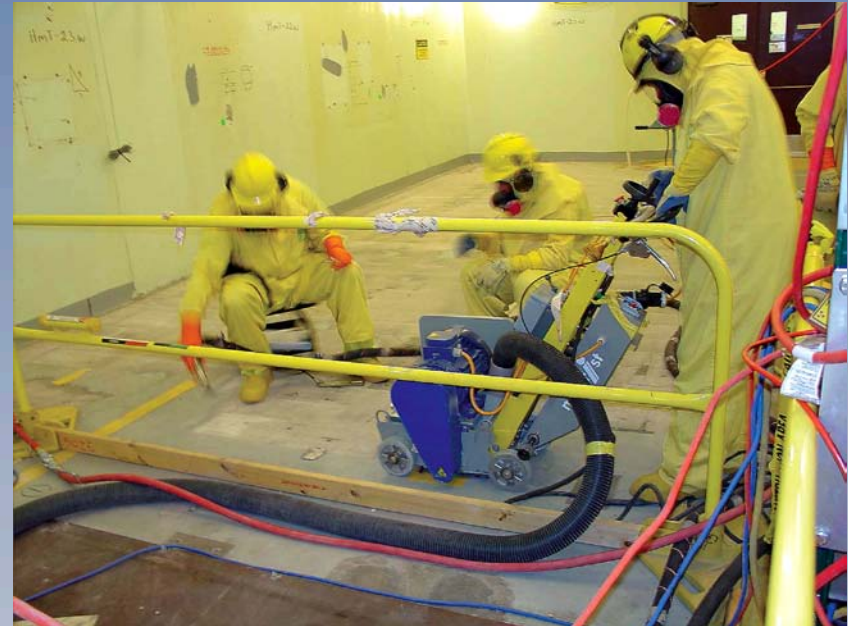
Floor Shaver removes contaminated concrete, allowing for ease of surveying / monitoring during decommissioning of Building 376 at Rocky Flats Nuclear Weapons Plant.
