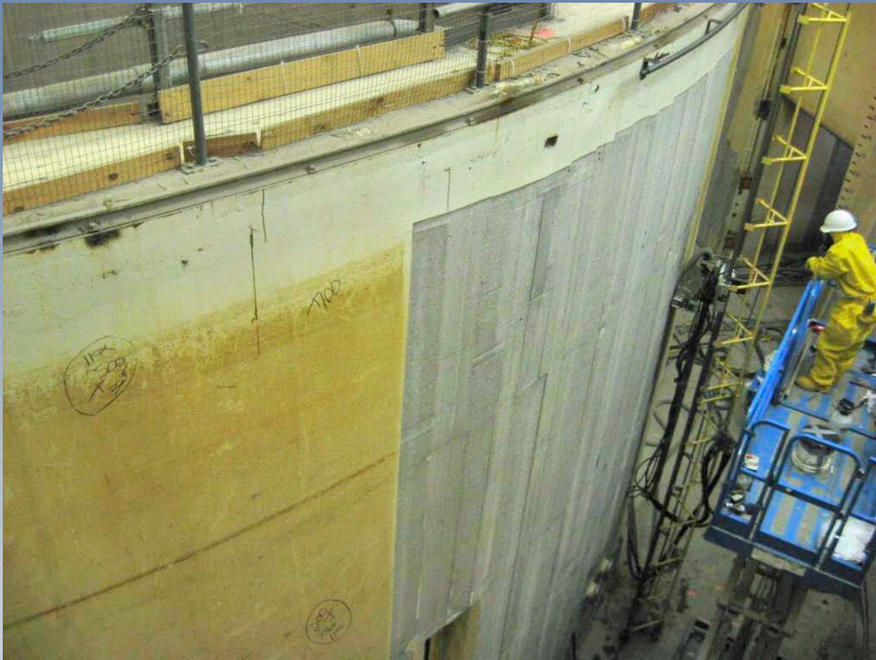
Diamond wall shavers with Bluegrass-engineered mountings removing contaminants from convex walls at Plum Brook Reactor Facility.
