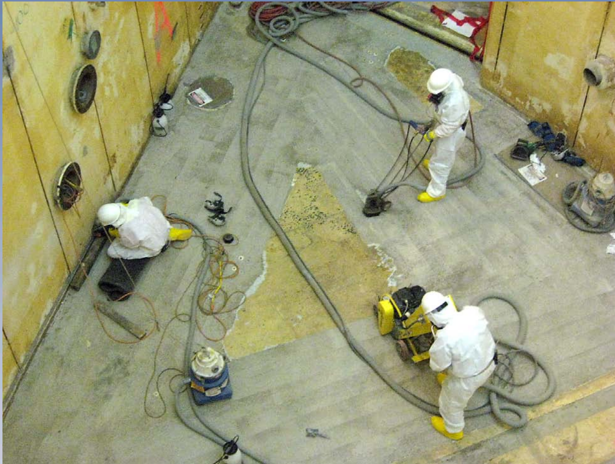
Diamond floor shavers being used to remove contaminants in Plum Brook Reactor decommissioning.
