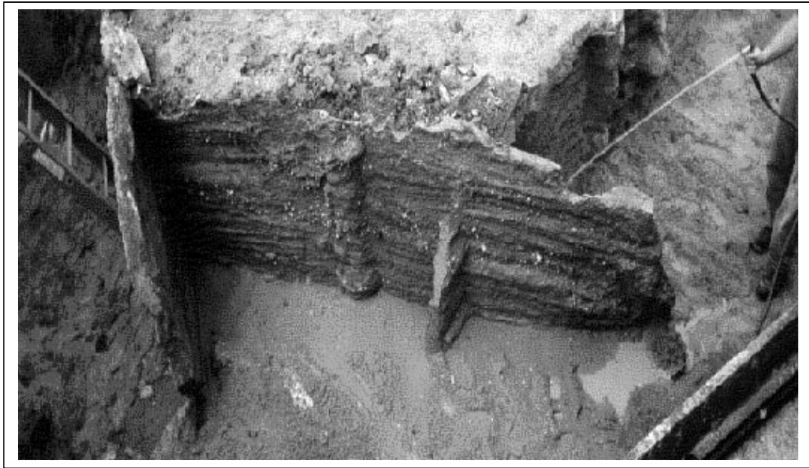
Figure 6. After examining three-dimensional ERT images at the Dover test site, a portion of a contaminant migration barrier was excavated for further evaluation. Electrical resistivity changes were imaged as salt water tracer moved through the barrier at locations later found to be defects in a wall or the joining of two walls.
