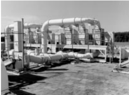
Figure 3. Exhaust System without Scaffolding
