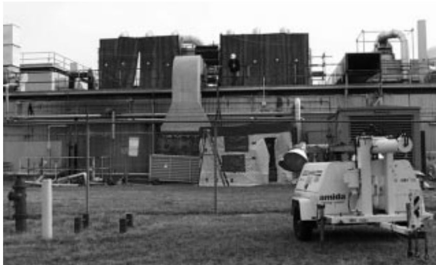
Figure 11. Portable Generator (foreground), Hut and Job Site Shielding (background)
