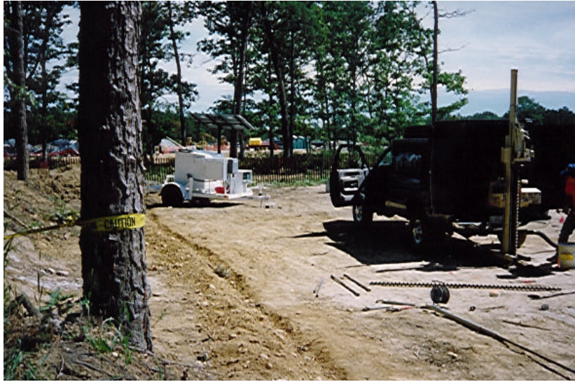
Figure 11. SEAttrace™ System remotely operated on site at the Viscous Liquid Barrier (VLB) test site in Brookhaven, NY (background). In the foreground, completion of the vapor sampling point installation can be seen.
