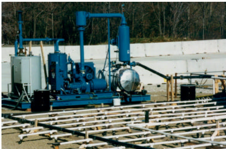
Figure 5. PVW field with extraction piping.
