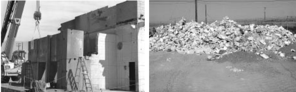
Figure 6. The Auxiliary Reactor Area-I D&D Site: hot cell demolition and cinderblock rubble for loading waste boxes and soft-sided containers.
