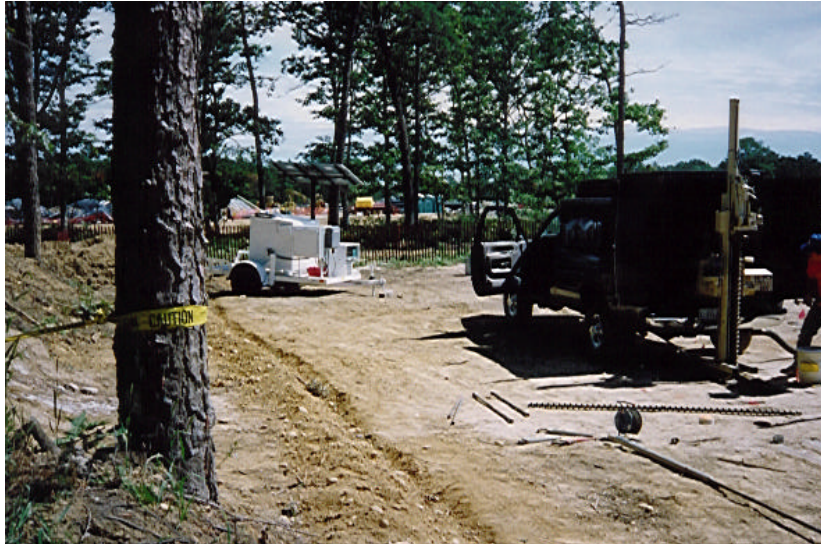
Figure 11. SEAttrace™ System remotely operated on site at the Viscous Liquid Barrier (VLB) test site in Brookhaven, NY (background). In the foreground, completion of the vapor sampling point installation can be seen.
