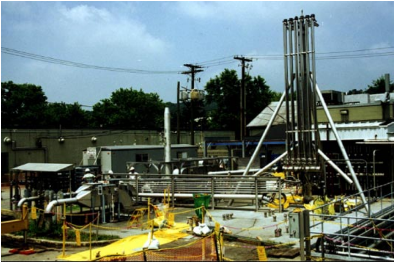
Figure 5. AEA Fluidic Pulse Jet Mixer deployed at the Bethel Valley Evaporator Storage Tanks site in Oak Ridge.
