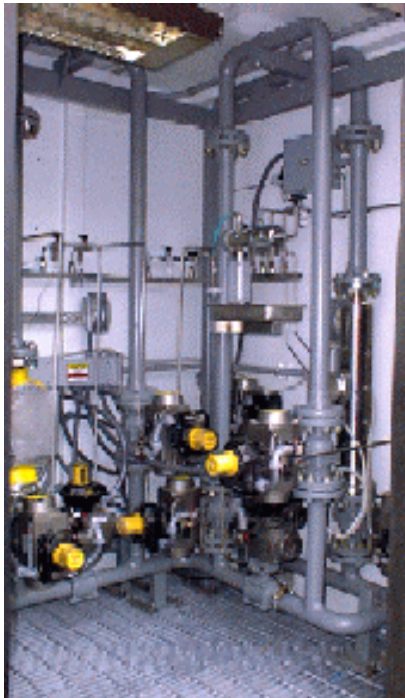
Figure 1. Endress+Hauser Promass 63M Coriolis meter installed in GAAT Slurry Monitoring Test Loop.
