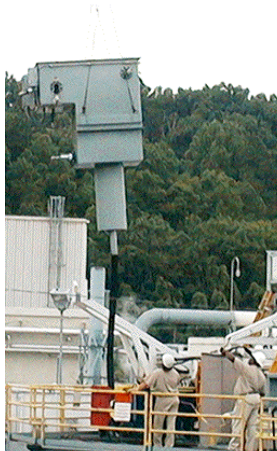
Figure 5. Waste Stream Consolidation System – surge tank during installation at Gunite and Associated Tanks Operable Unit, Tank W-9.
