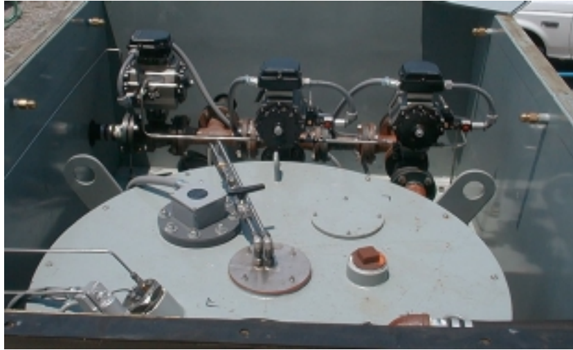
Figure 6. Waste Stream Consolidation System – surge tank top view, inside secondary containment.
