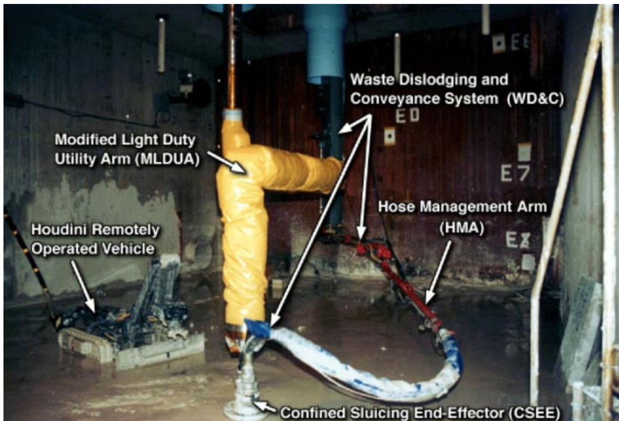
Figure 12. GAAT retrieval equipment in the ORNL Tanks Technology Cold-Test Facility.
