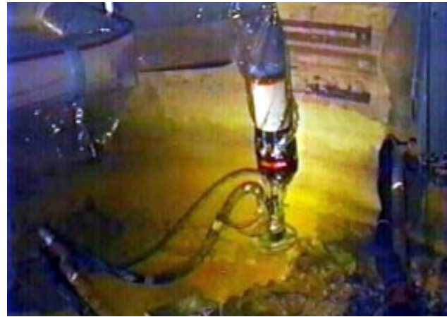
Figure 11. MLDUA being used to deploy the confined sluicing end effector in an ORNL gunite tank.
