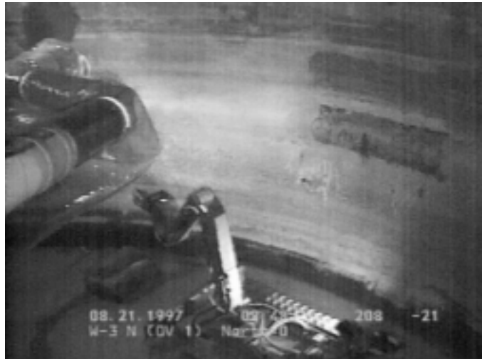
Figure 18- The Modified Light Duty Utility Arm (MLDUA) and Houdini at work at ORNL
