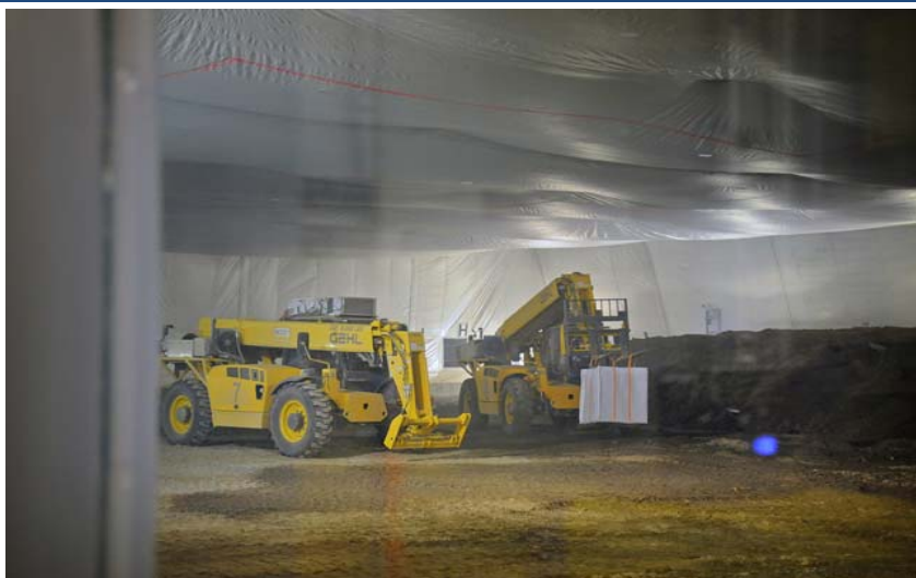
Waste exhumation underway at the Idaho Cleanup Project executed under ARRA (Reference 2).
