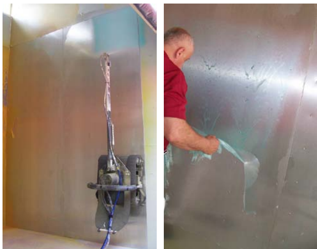
Integrated remote spraying platform - scaling up a vertical wall in building module and applying DeconGel to metal panel. Dry DeconGel peeling from metal panel.
