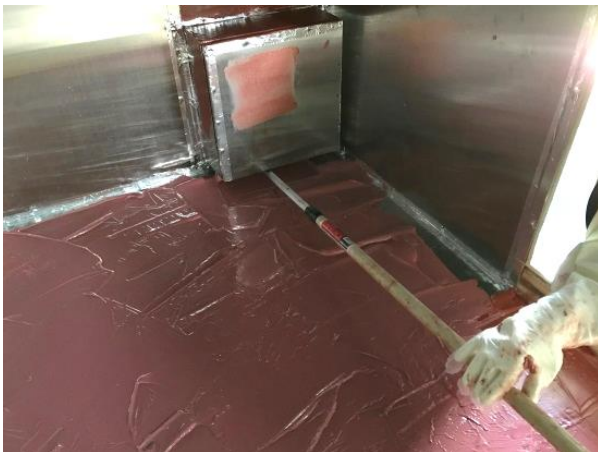
Application of IC technology simulating operational conditions at the FIU Hot Cell Test Bed Facility
